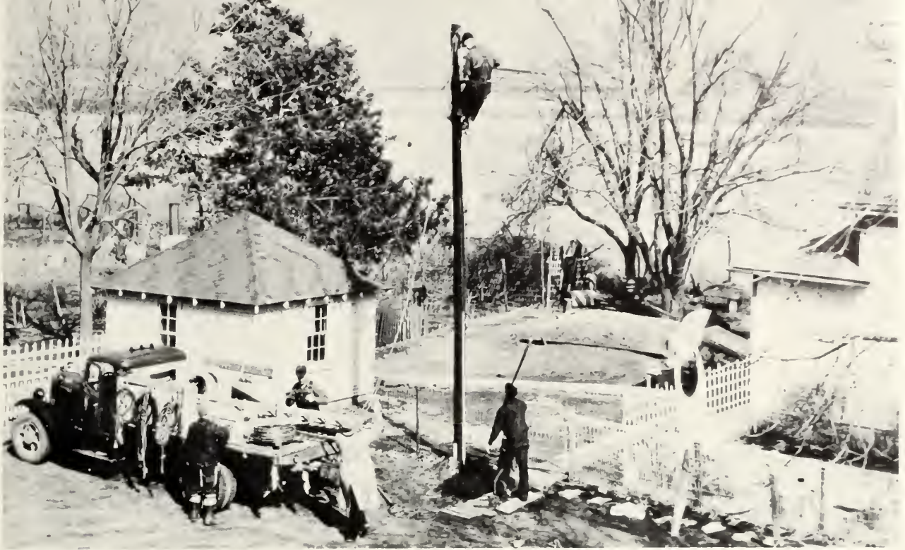
Considerable planning went into the placement of poles. If a windstorm was to topple this one, it would not strike the building. Note storm cellar behind house.
